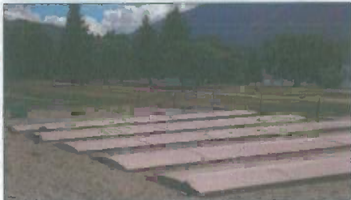
This array of AX-Max units provides wastewater treatment for a large resort and camping area in New Zealand.
